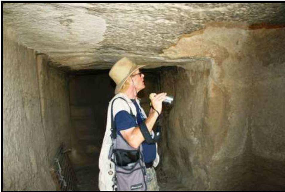
The author inspecting the water weathering in level 2
